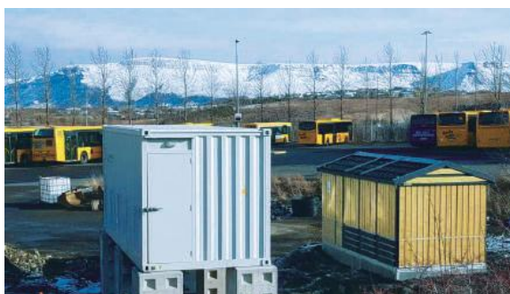
Pure electric bus charging project in Reykjavik, Iceland
